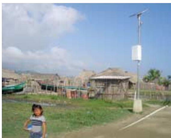
Figure 7–2 An example of the photovoltaic systems installed in the Kuna Indian community of Ustupu in Panama. The community has a population of 4,000. (Photo: Markku Nurmi)
